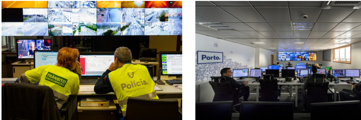
Integrated Management Center (CGI) of the Municipality of Porto in 2015 (left) and 2016 (right).
