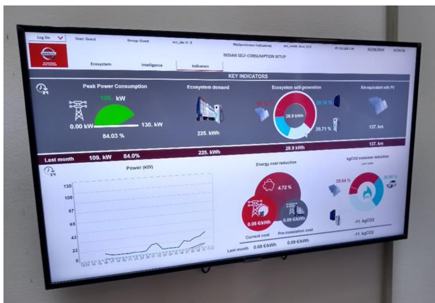
Figure 217 TV SCADA screen in Nissan offices
