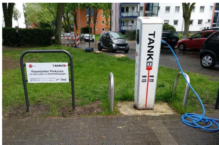
Figure 206 Stegerwaldsiedlung charging station (M11.1 Cologne)
