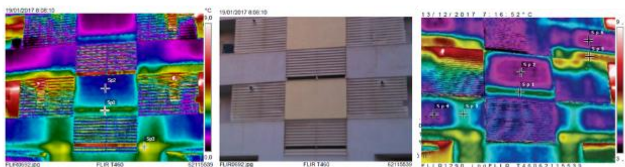
Figure 76 Thermal image of south facade before (left) and after (right) facade thermal upgrade works
