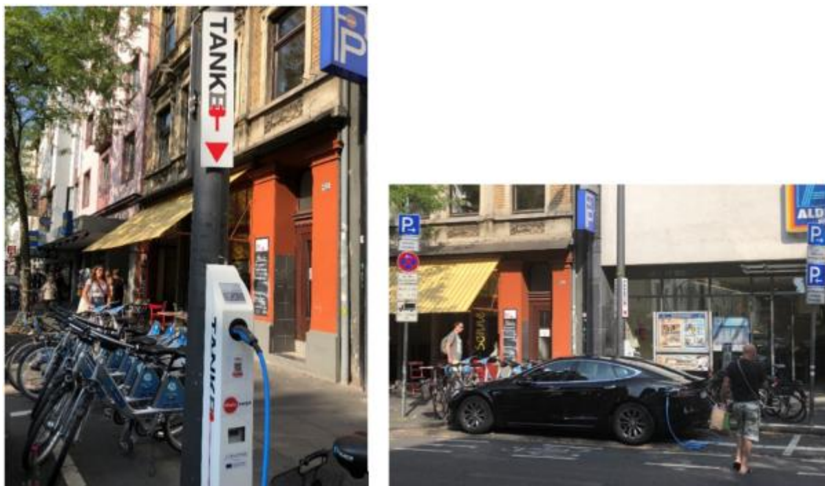
Figure 127 Charging stations installed in Cologne
