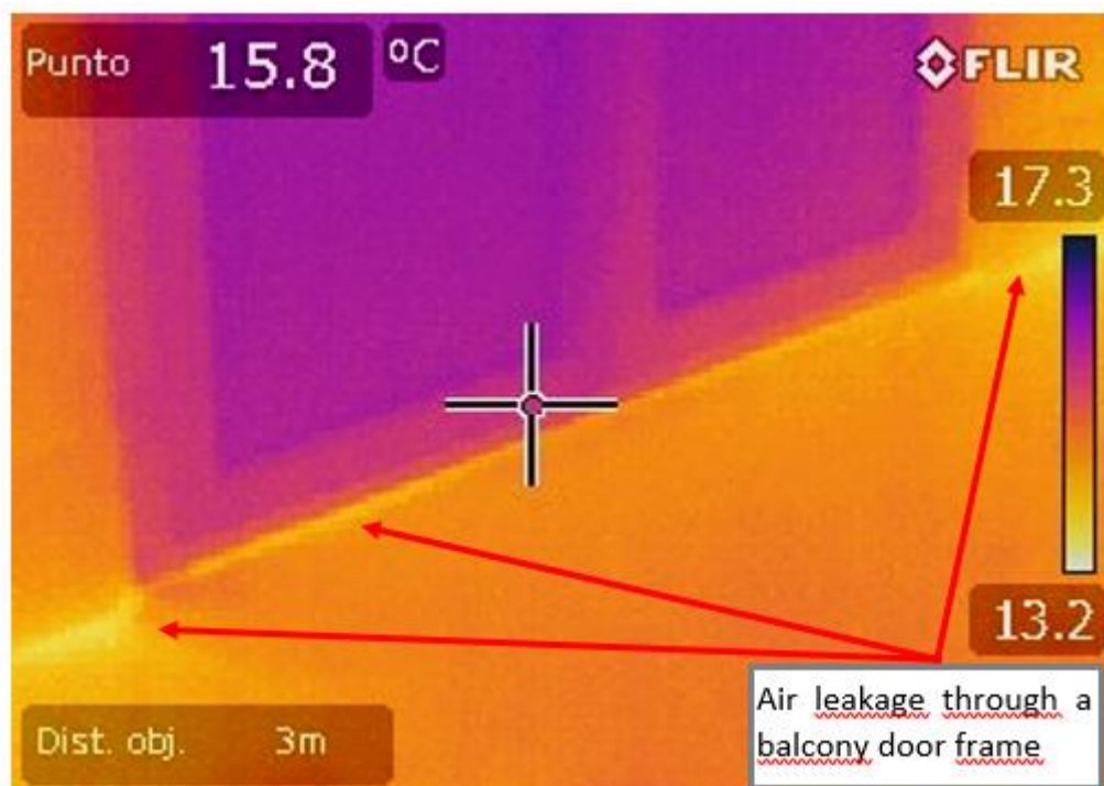
Figure 83 H10 Madison: thermal imaging after the refurbishment (poor installation)
