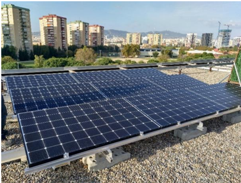
Figure 211 PV system at Nissan office
