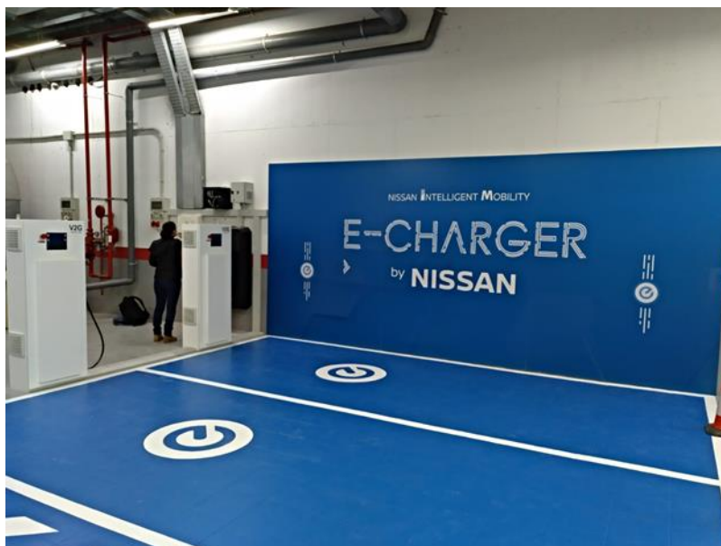
Figure 212 V2G chargers at Nissan office
