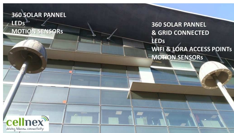
Solar HUB for communications system
